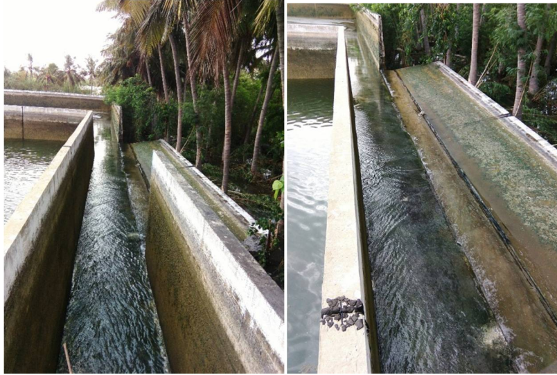
Figure 1 : Collapsed Ground level reservoir Photos
