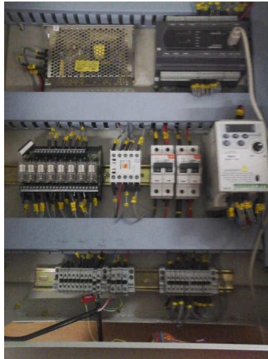
Fig 3.: PLC Panel Board
