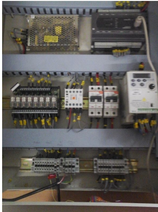
Fig 3.: PLC Panel Board
