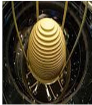
Fig: 4 Tuned mass Damper
