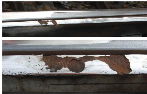
Fig 2: squats on railway track
