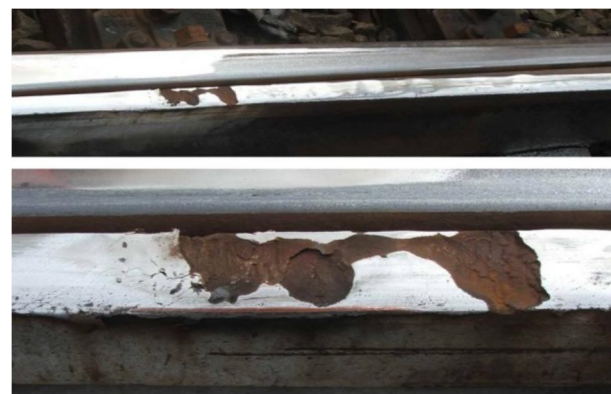
Fig 2: squats on railway track
