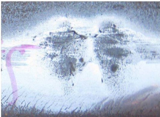
Fig 1: squats in railway track
