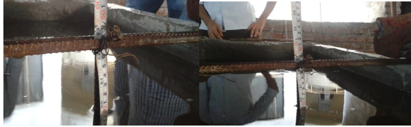
Photo-measurements of depth of leakage
