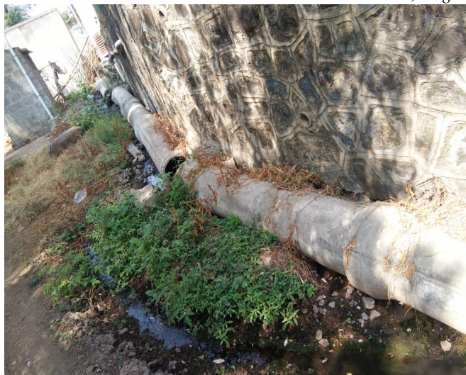
Fig.2 Poor Sewage Disposal System in kondave village
