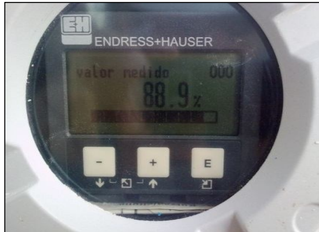
Fig. 15 Radar FC-LT-509 Installed.
