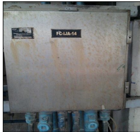
Fig. 9 Junction Box (FF-IJA-14)
