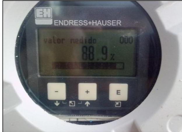
Fig. 15 Radar FC-LT-509 Installed.
