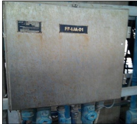
Fig. 6. Junction Box (FF-IJA-01)
