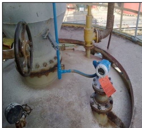
Fig 14. Radar FC-LT-510 installed.
