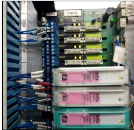
Fig. 12 Cabinet Interior View – SIH
