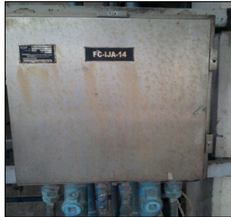
Fig. 9 Junction Box (FF-IJA-14)
