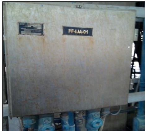
Fig. 6. Junction Box (FF-IJA-01)
