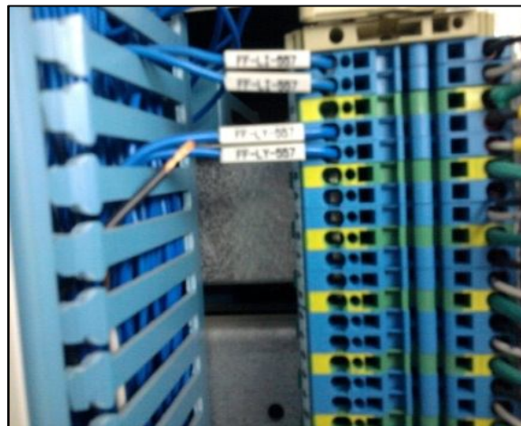
Fig. 11 Terminal block. Arrival of Radar Threads
