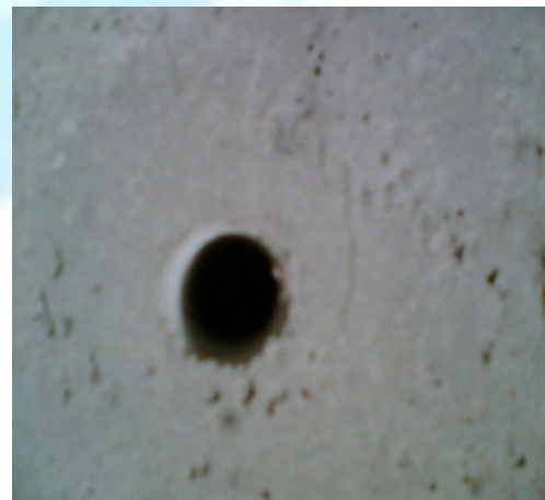
Fig. Hole in the brick
